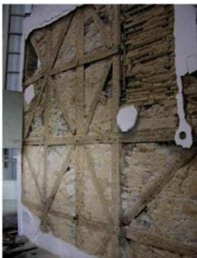
Fig 2.12: Gaiola Wall after Test
