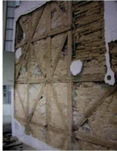
Fig 2.81: Gaiola Wall after Test
