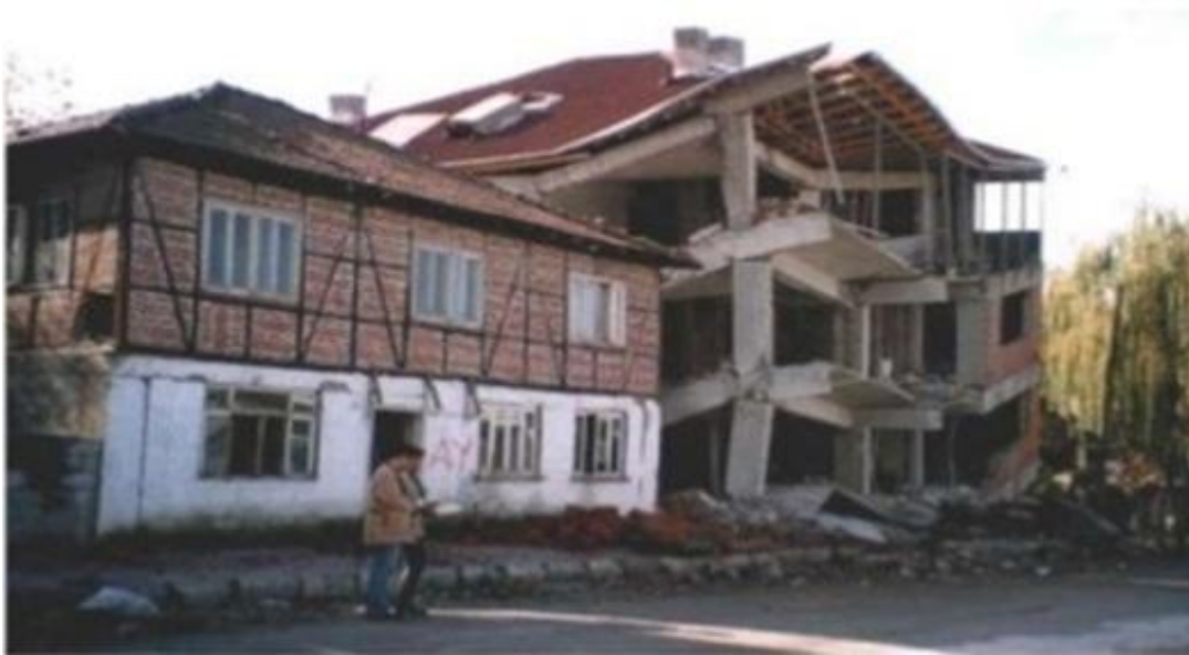
Fig 2.10: An Example of (1999) Turkey Earthquake [16]
