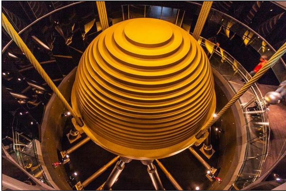
Figure 1.3: Taipei 101 Tuned mass damper
