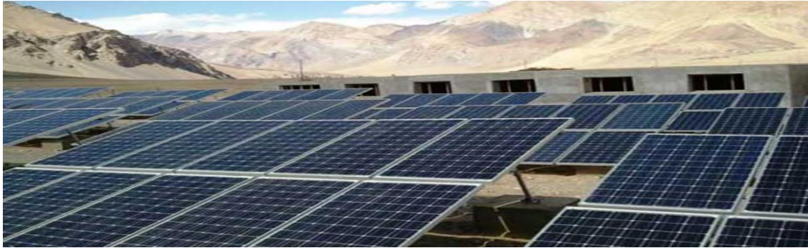
Figure 2.13 Leh and Kargil Solar Power Projects [35]
