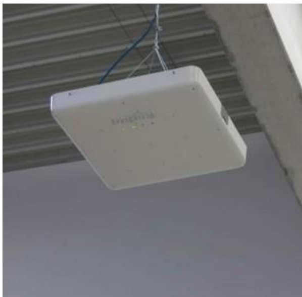
Figure 5-2: An overhead Antenna
