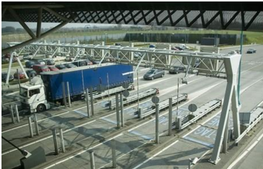
Figure 5-4: Light Curtains installed at a toll station
