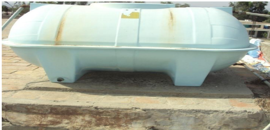
Figure 6.2: Water Tank on Event's Hall Roof
