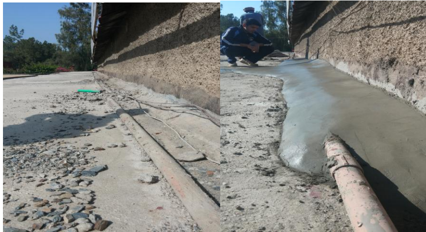
Figure 6.3: Subject Seepage Place and its treatment
