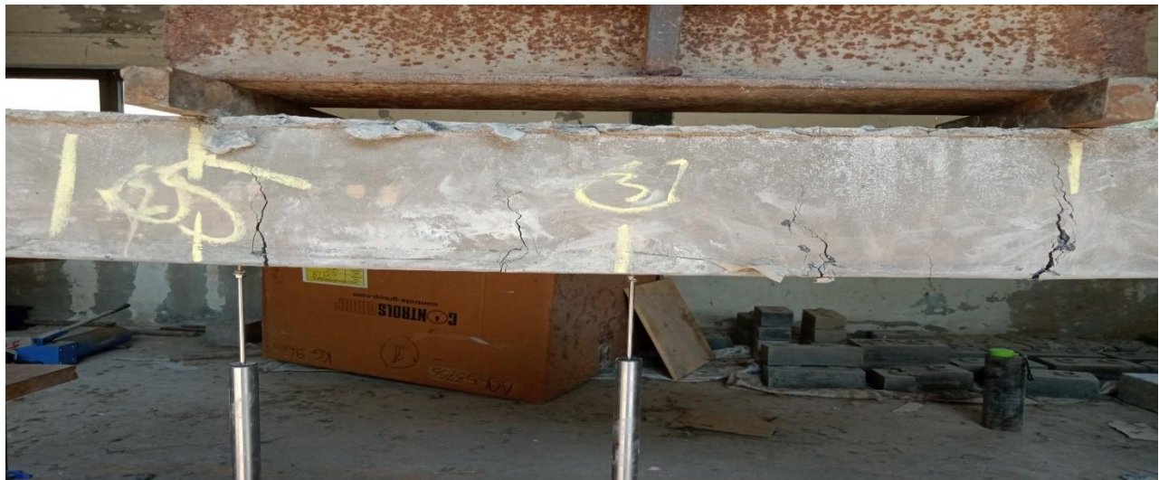
Figure 4.15: Failure pattern of beam with flexural and steel fibers reinforcement (SF-R)
