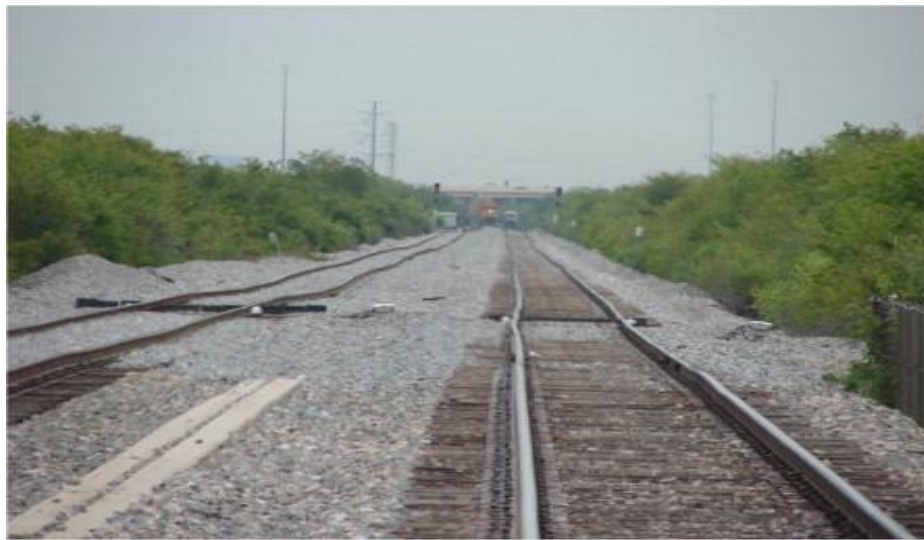
Figure 1.2 Cracks in Lightweight Structures (Railroads)
