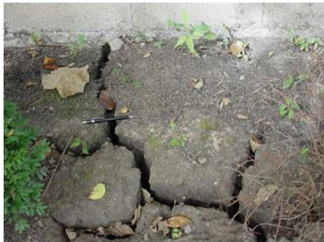
Figure 1. 5 Cracks in expansive soil
