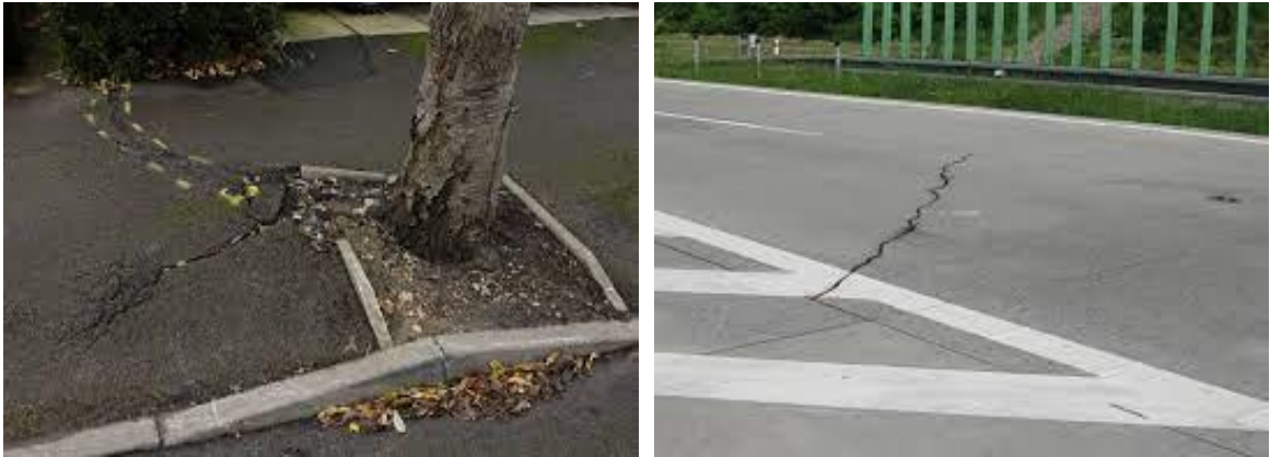
Figure 1.3 Cracks in Lightweight Structures (Roads)
