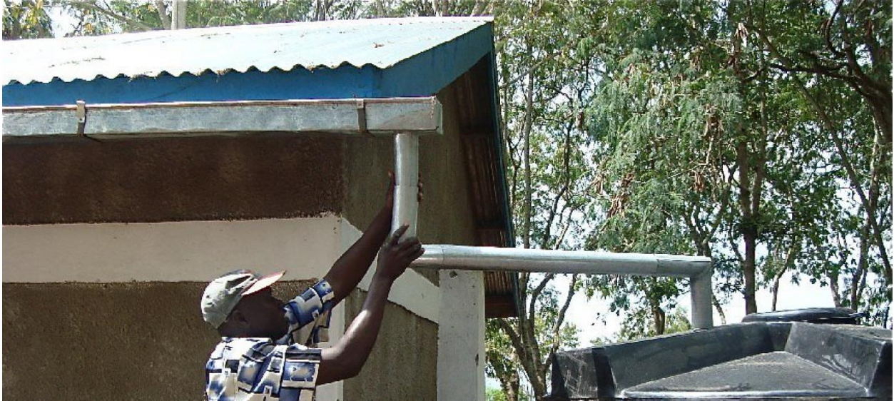
Fig 5.6 Roof water harvesting
