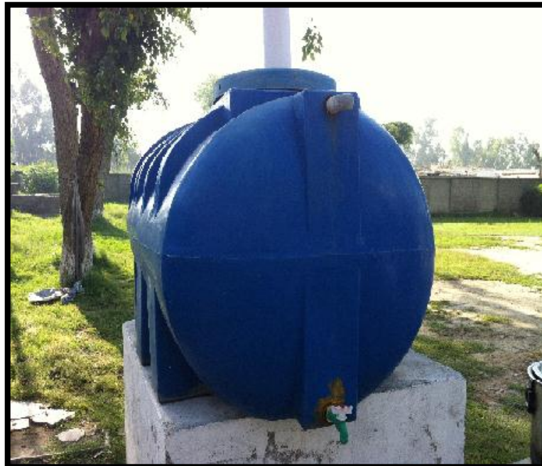
Fig 7.5 Fiber Glass Water Tank
