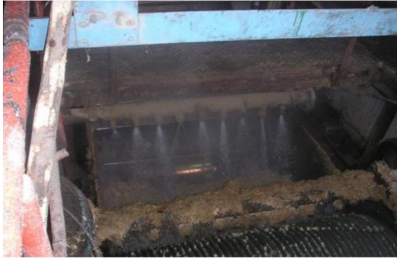
Figure 4.1: Feed water sprinkling in Mill
