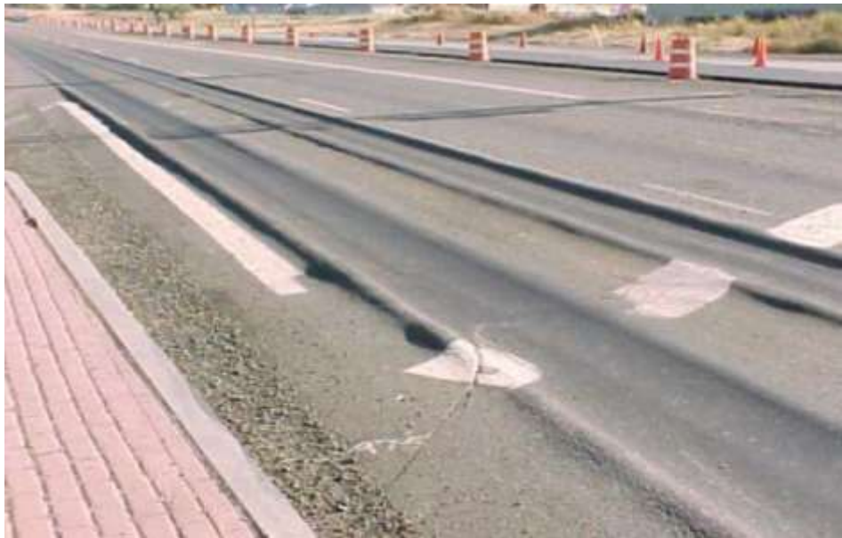
Figure 2.1. Pavement appearance constructed on expansive soil subgrade
