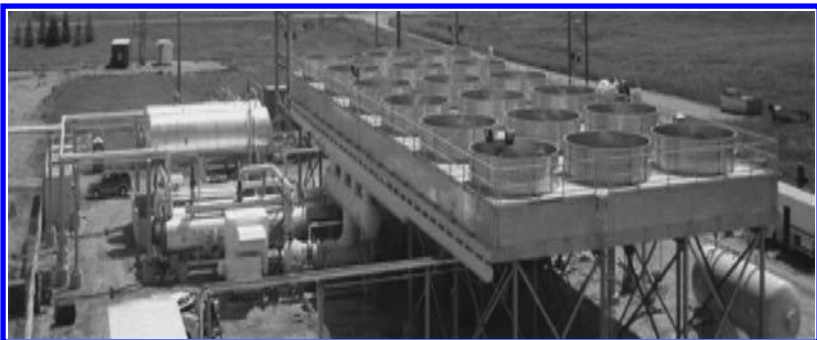
FIGURE 3.1 Air cooling system for wastewater from SAGD system, Alberta, Canada.
