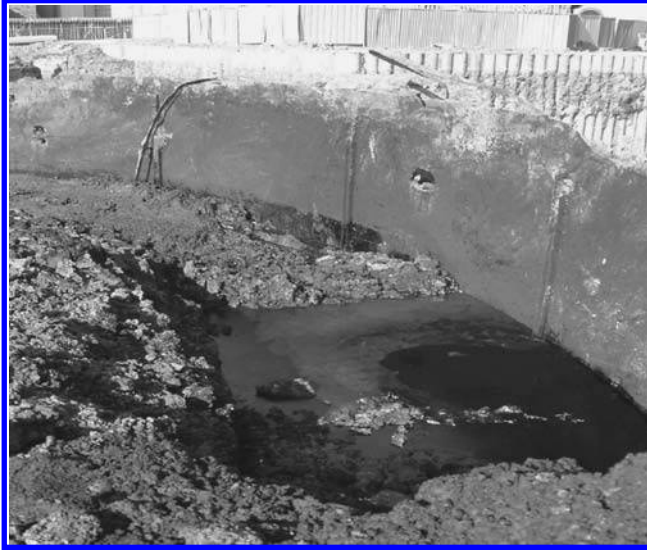
FIGURE 7.6 Photo of coal tar in excavation at an MGP site during remediation. In this case, the NAPL is contained within an old gas holder base.
