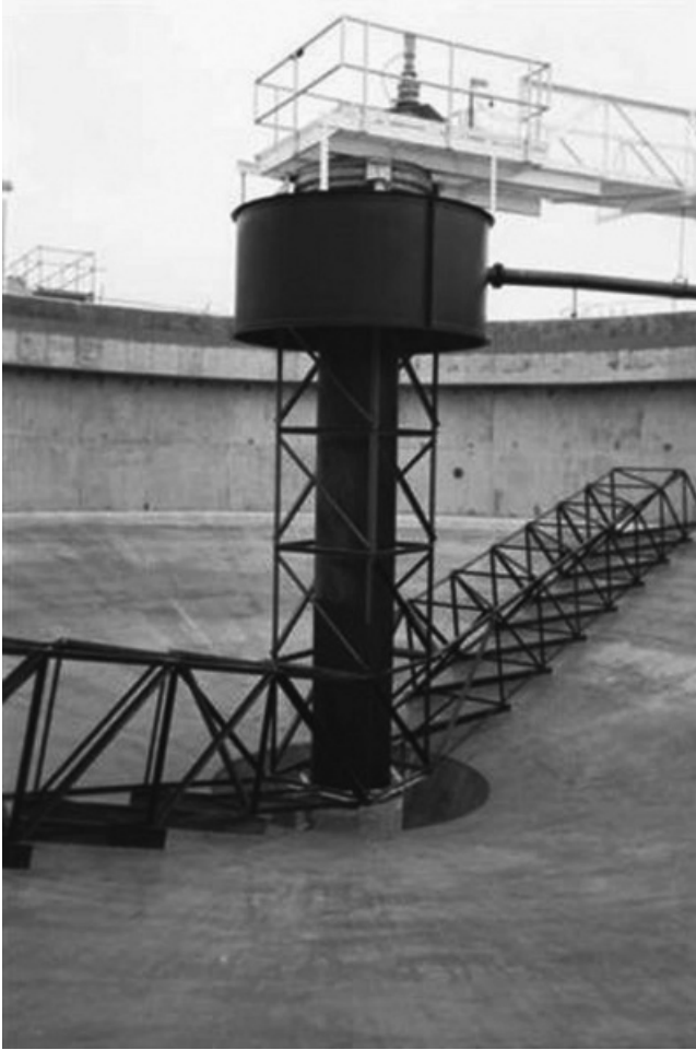
FIGURE 7.4 Innards of a sludge thickener. Note steeply sloping sides and mechanical rake which promotes sludge compaction & collection in the center well. Other manufacturers will have tanks with steeper sides and vertical poles (rakes) on the collector mechanism to promote thickening. Photo courtesy Wes-Tech Engineering Salt Lake City, UT.
