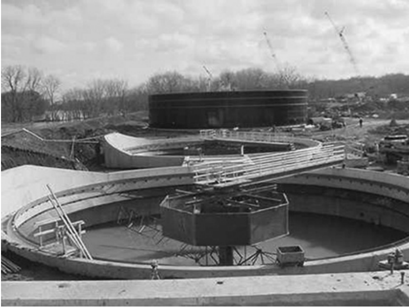
FIGURE 7.3 Circular clarifier under construction—Observed the center baffle that is used to direct the flow downward, under the baffle, before the flow flows outward to the launder ring (scum and floatable barrier) and the overflow weir around the periphery. Source: Greeley and Hansen-Lafayette, Ind.
