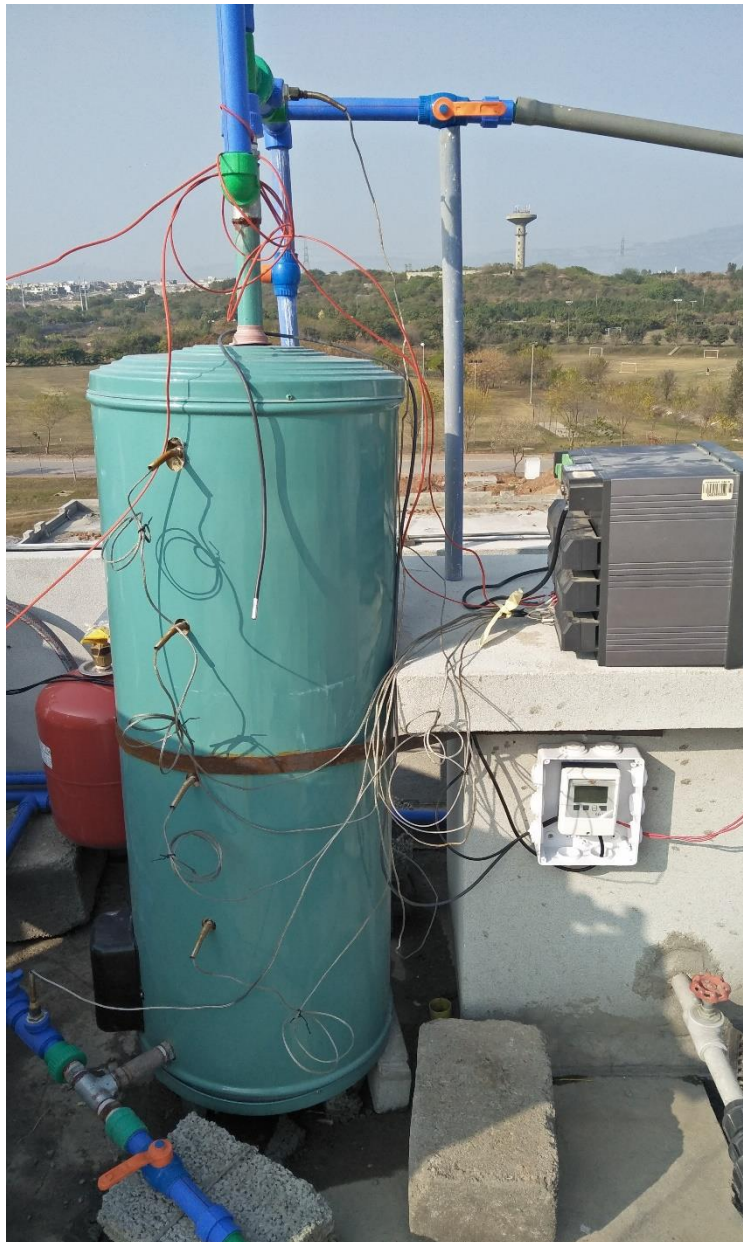
Figure 3.4 Storage tank installed as a heat exchanger for hot water system
