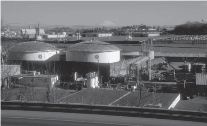
Storage tanks with secondary containment
