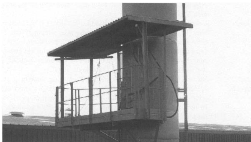
Figure 5.12 Sampling platform (courtesy of SGL Technic Ltd)
