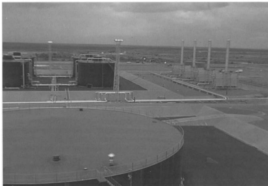
Figure 10.15 Venting system for crude oil storage tanks, Oritupano-Leona, Venezuela (courtesy of Cordah Limited and Perez Companc SA)
