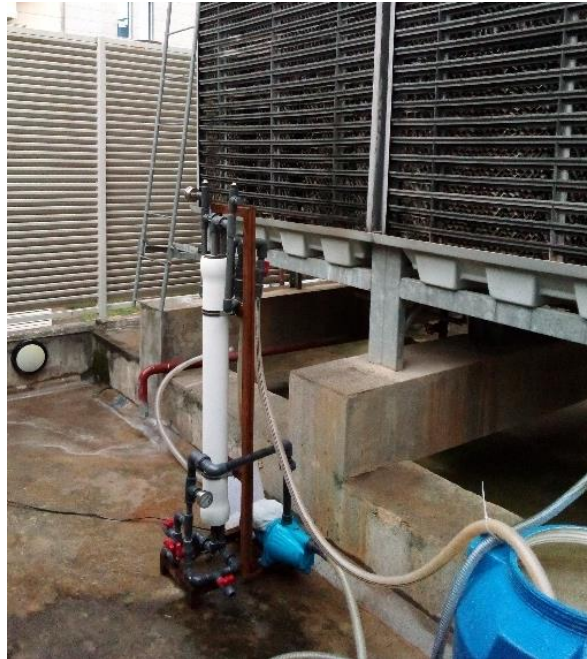
Figure 17: Recycled Membrane filtration at Cooling Tower Blowdown water
