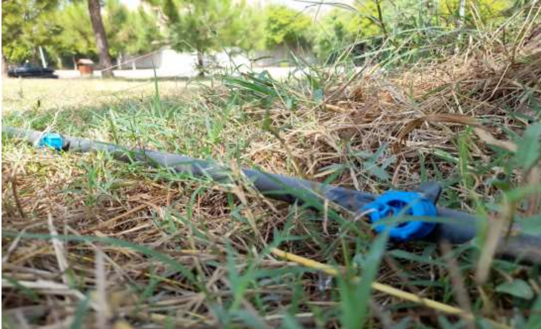
Figure 2-2 Drip Irrigation system Installed at NBS Lawn NUST
