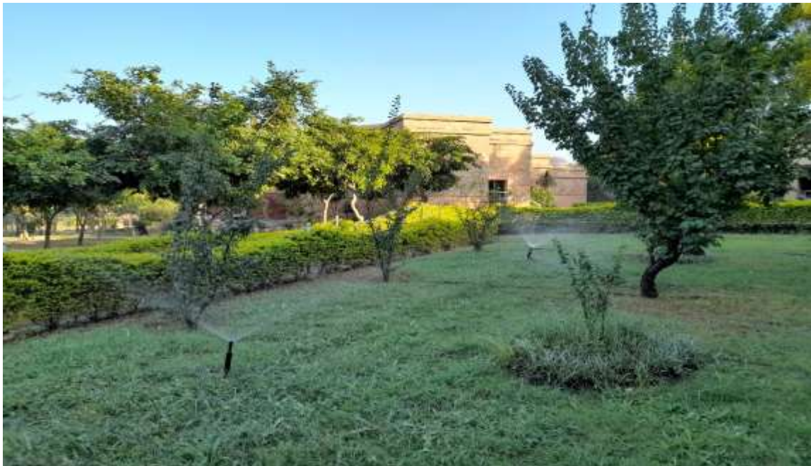
Figure 2-1 Sprinkler's Installed at NBS Lawn NUST.
