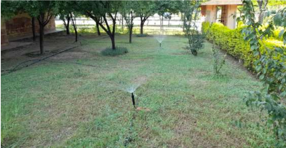
Figure 3-5 Six type of Sprinklers installed at NBS Lawn.
