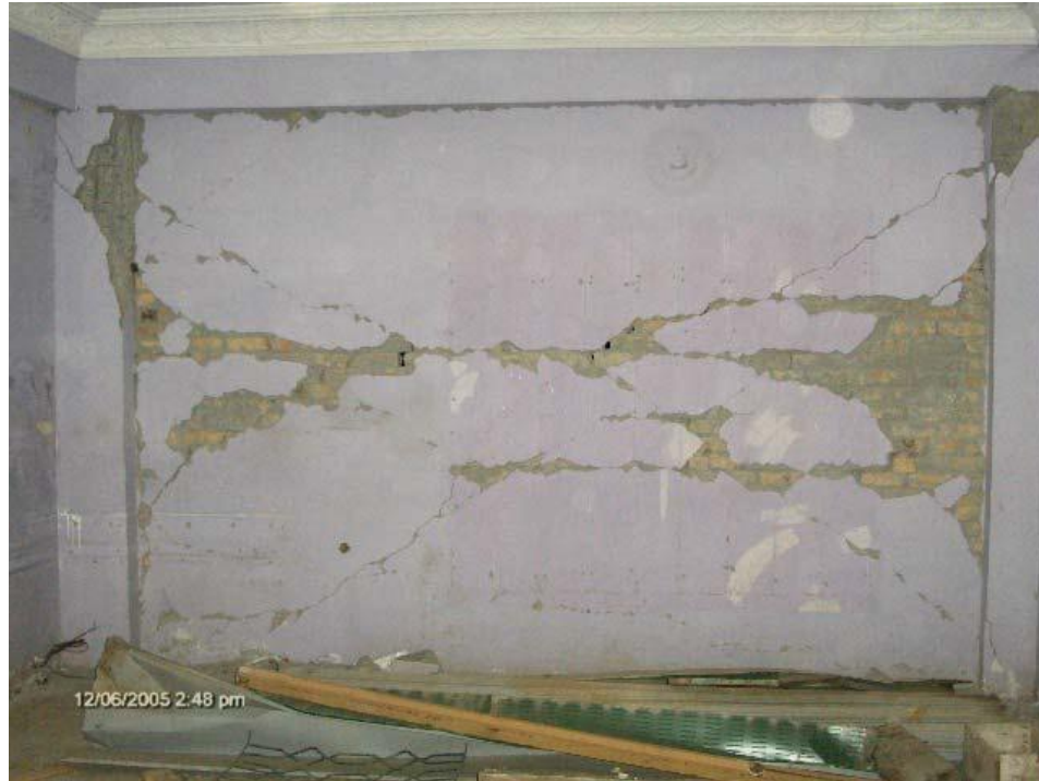
Figure 1.1: Failure of masonry infill walls due to the diagonal compressive forces transferred from column-beam joint, during Kashmir (2005) earthquake (Javed, 2009).
