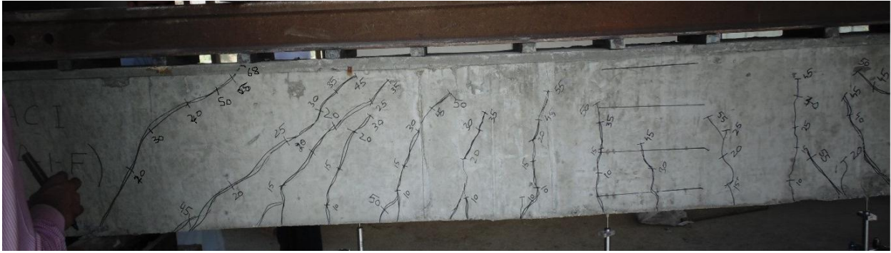
4-10: Cracked Pattern of ACI-I
