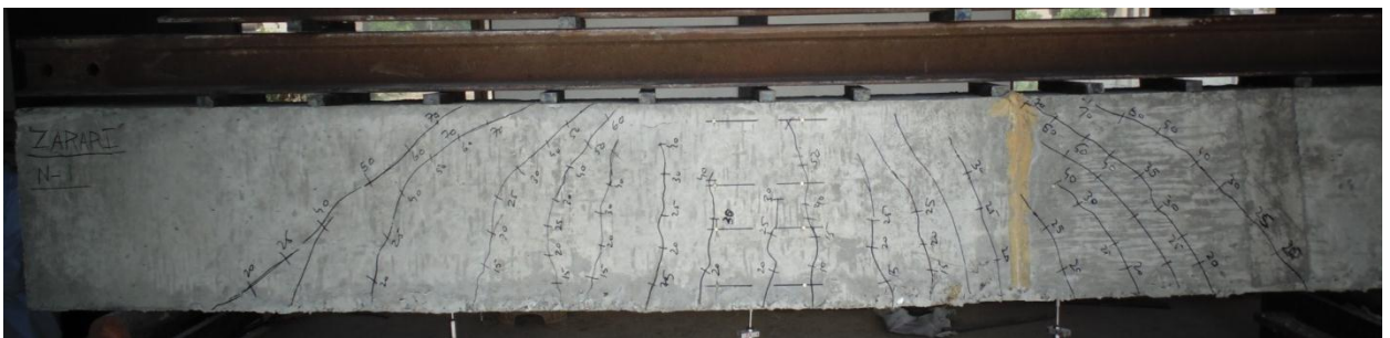
Figure 4-14: Cracked Pattern of Z-I
