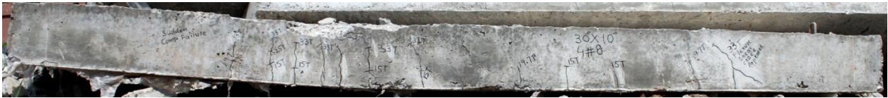
Fig4.4 Cracking pattern of W1
