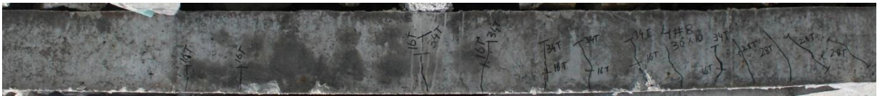
Fig4.8 Cracking pattern of W2
