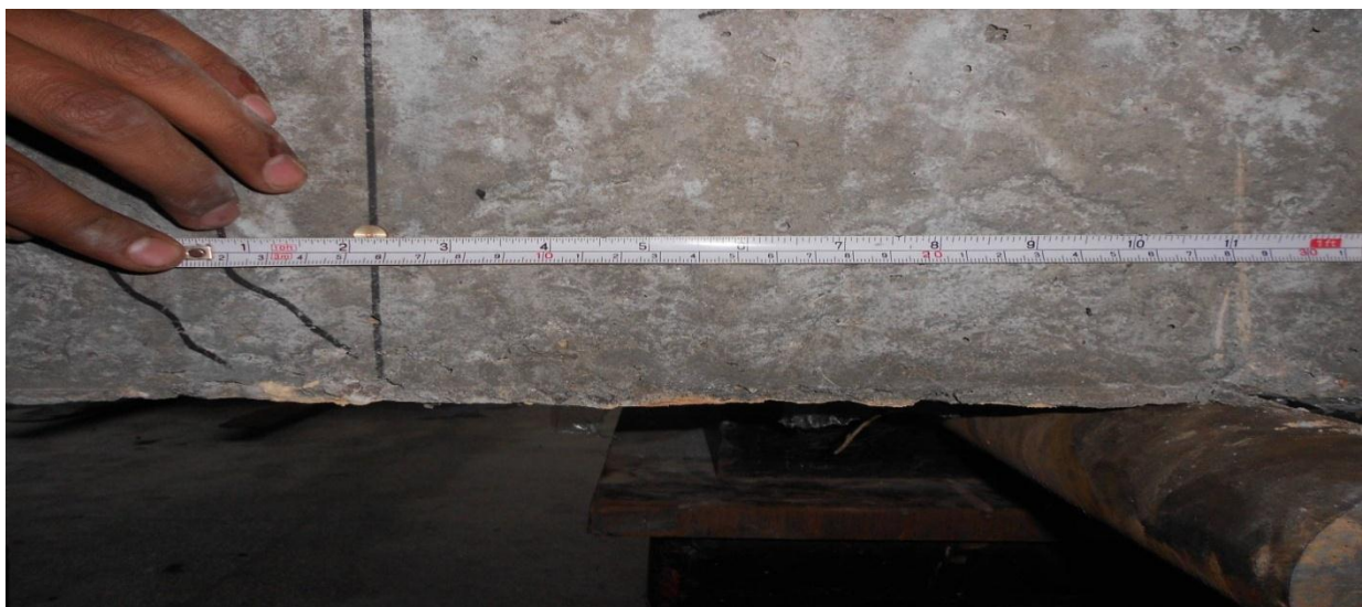
Fig4.13 Picture showing distance of shear crack from center of support
