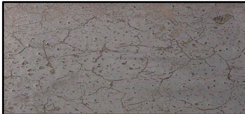
Fig.4.1 A concrete slab showing cracks due to excessive water in mix [5]
