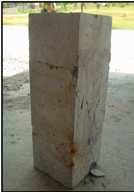
Fig.3.6 A PCC Repaired Column after failure
