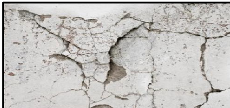
Fig. 4.2 A Concrete member showing cracks due to freezing and thawing [6]
