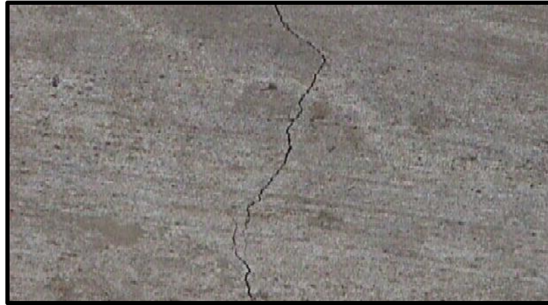
Fig. 4.7 A Crack in a concrete member due to structural overload [5]
