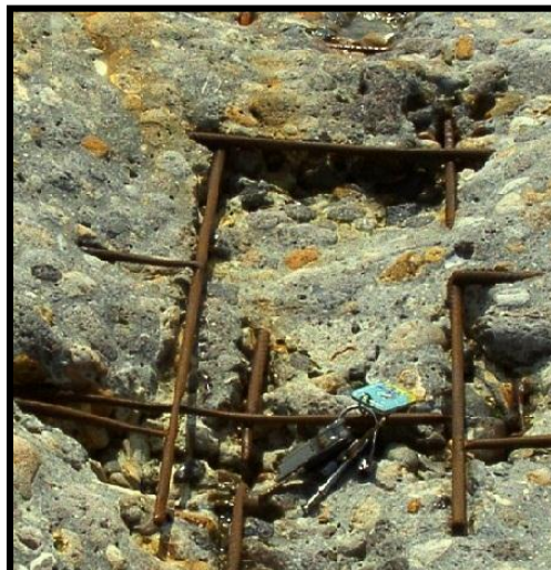
Fig. 4.4 A Concrete member erosion with exposed reinforcement [9]
