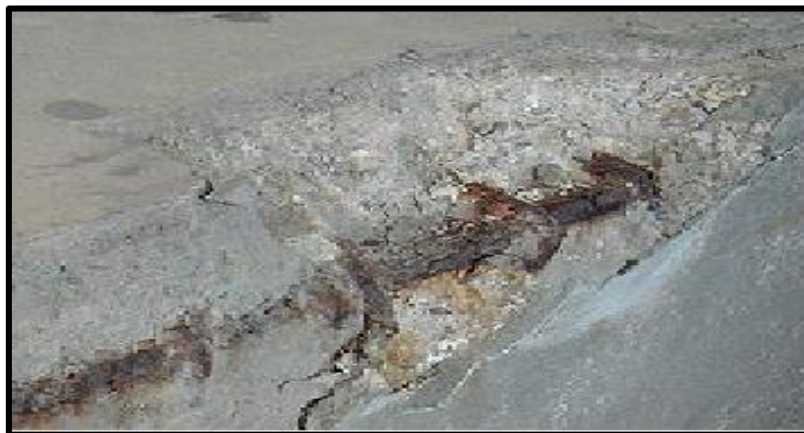
Fig. 4.6 A concrete member damaged due to acid attack [7]
