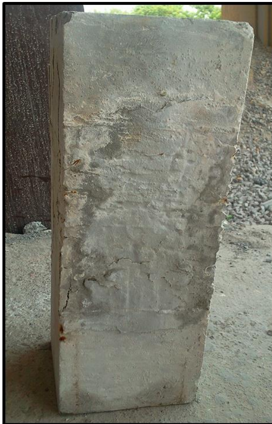
Fig. 3.7 A FRC Repaired Column after failure
