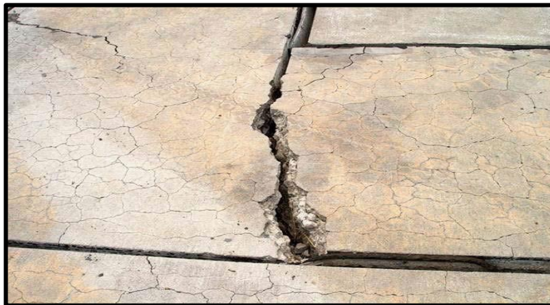
Fig. 4.8 A Crack in a concrete member due to High impact loads [5]
