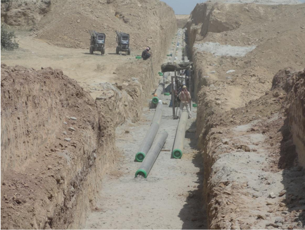
Figure 7: Package 6: (Hydrant refueling system) Trenches being excavated to lay the pipeline for providing fuel to the aircraft.
