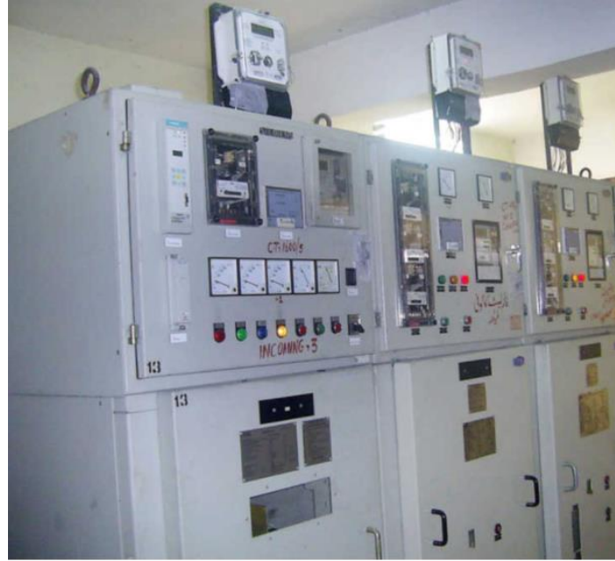
Figure 2-3. Energy sensors installed on circuits in one grid station.
