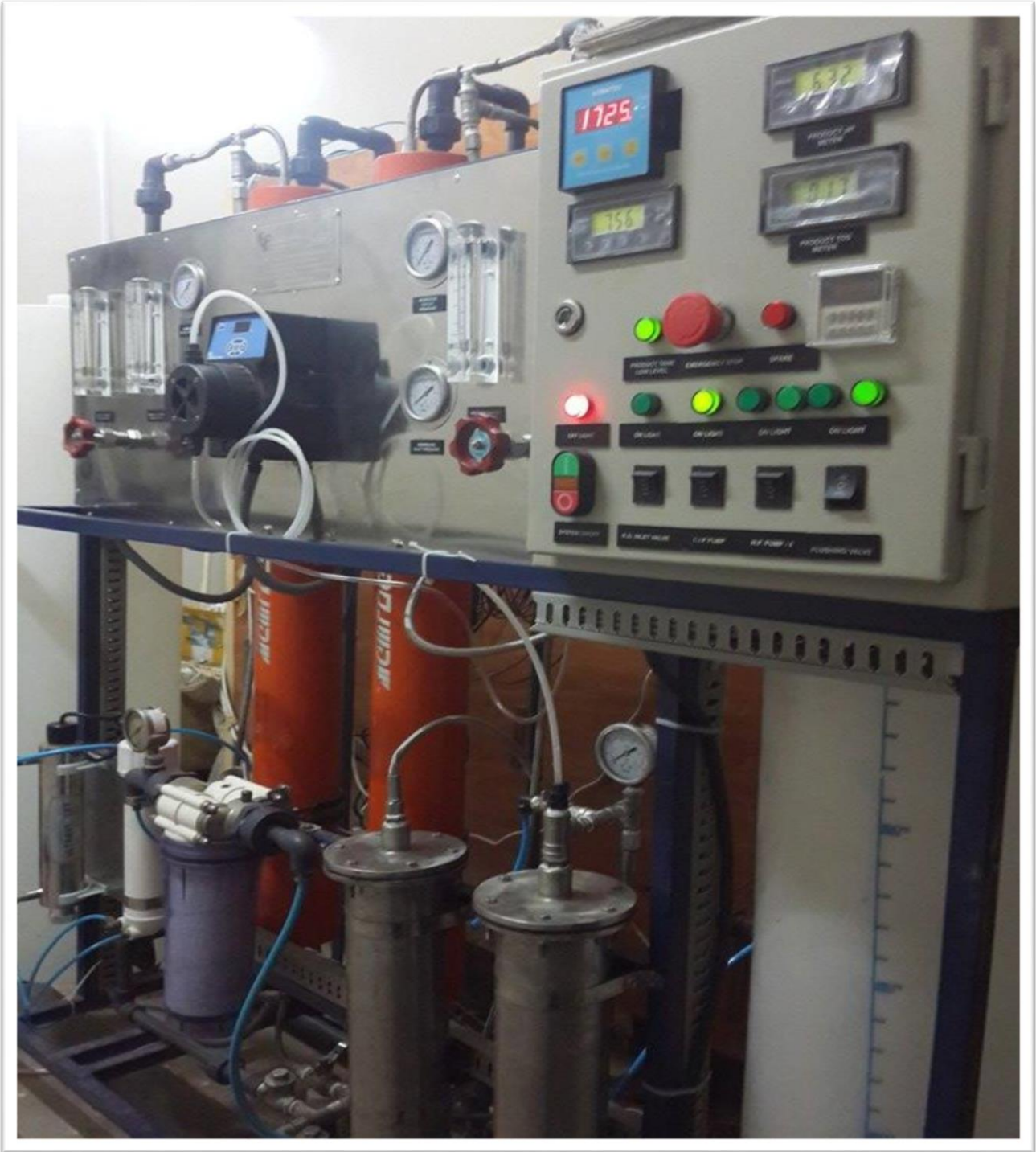
Figure 3.2: Pilot-Scale Reverse Osmosis Plant
