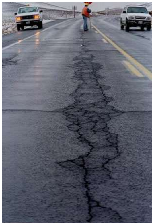
Figure 2.2: Pavement with moisture damage
