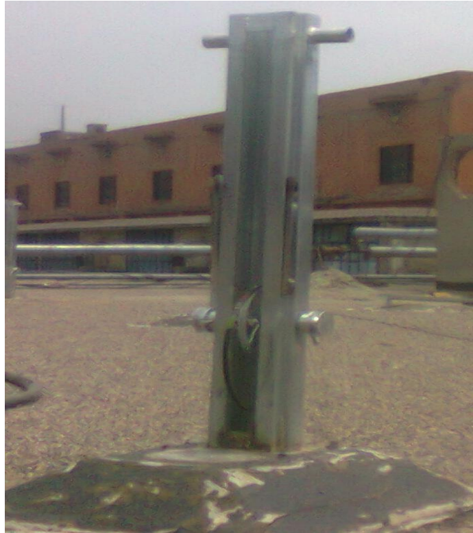
Fig. 4. 9 The stand on which trough is hanged fixed and level by concrete
