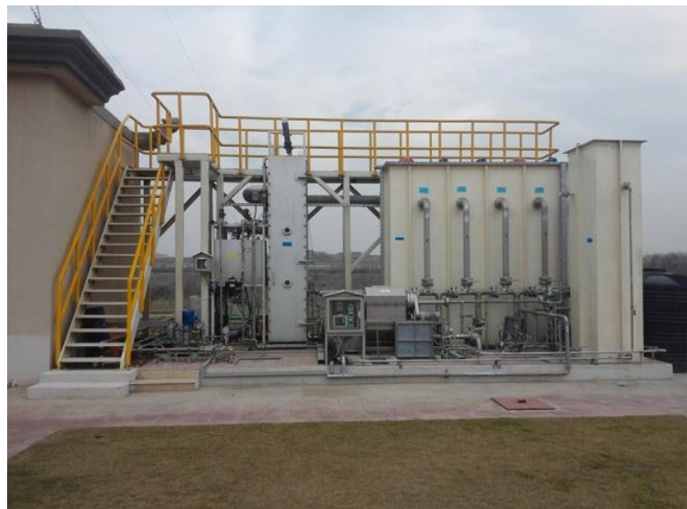
Fig. 1. NUST MBR plant
