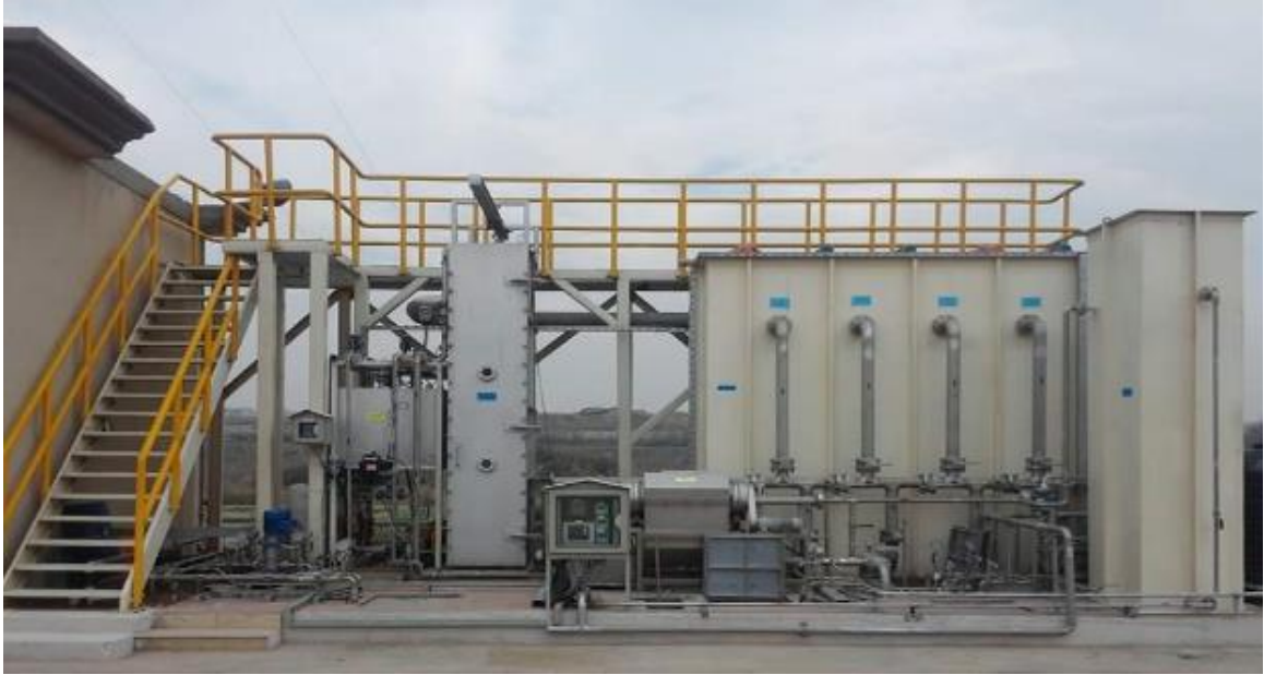
Figure 9: Actual Pictorial view of Full Scale MBR Plant
