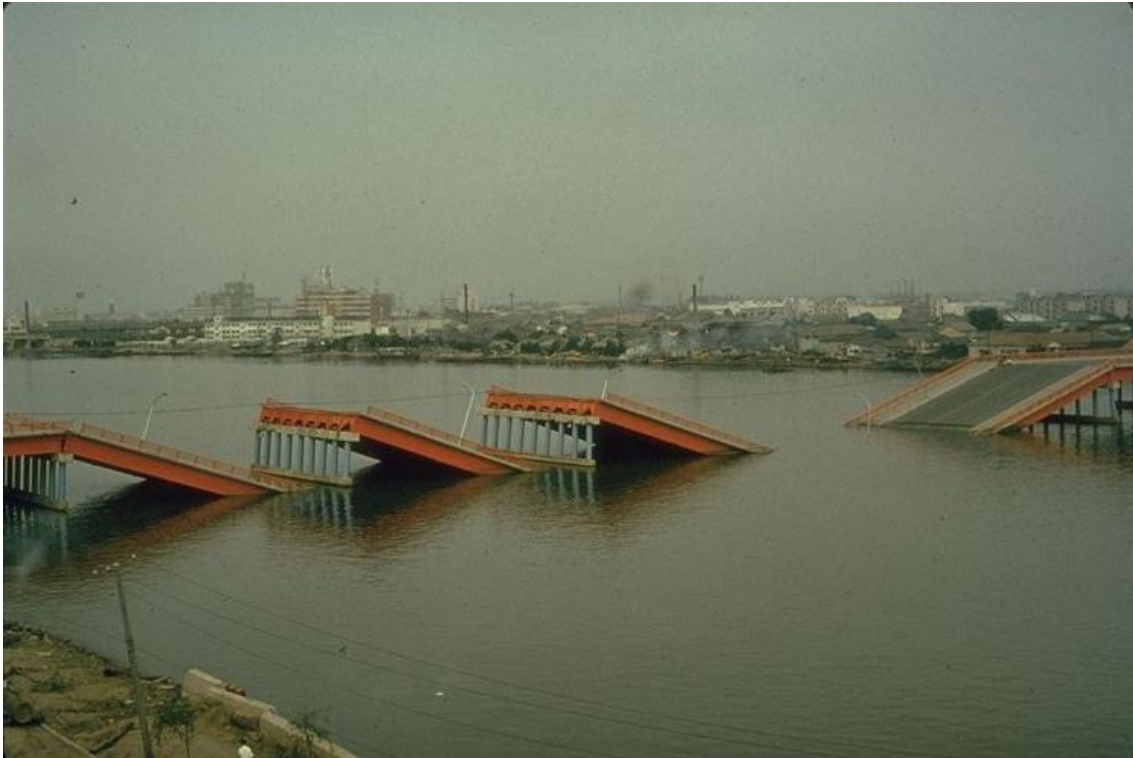
Figure 11.8 Lateral Spreading causing bridge spans to fall off from its supports, 1964, Niigata Japan
