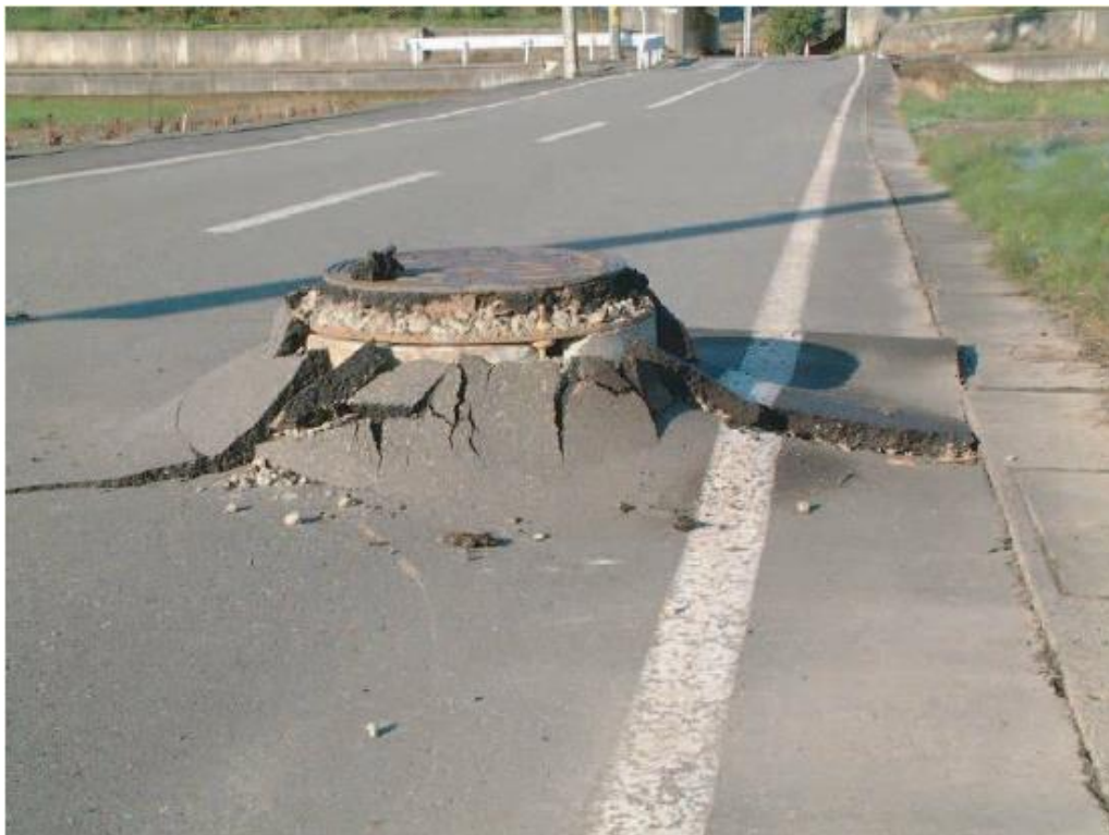
Figure 4.1 Uplifted buried structures after 2004 Niigata Chuetsu, Japan
