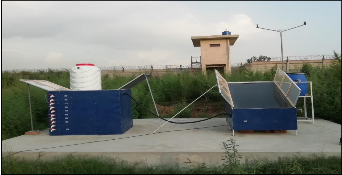
Figure 9. Treatment Unit near NUST MBR Plant
