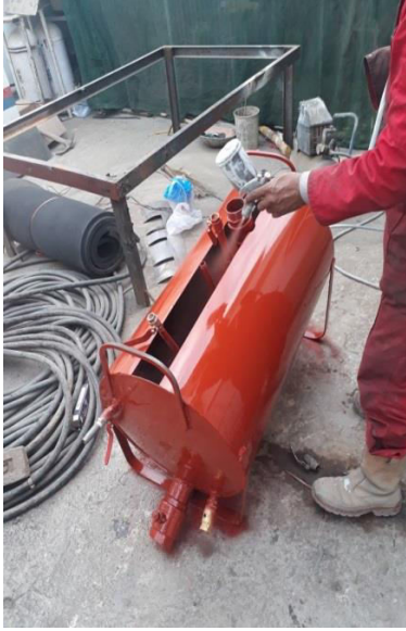
Figure 22 Lead Oxide coating on reactor outer body
