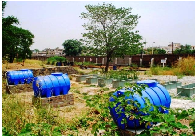
Figure.3.2. Pumps supplying refinery wastewater to containers.
