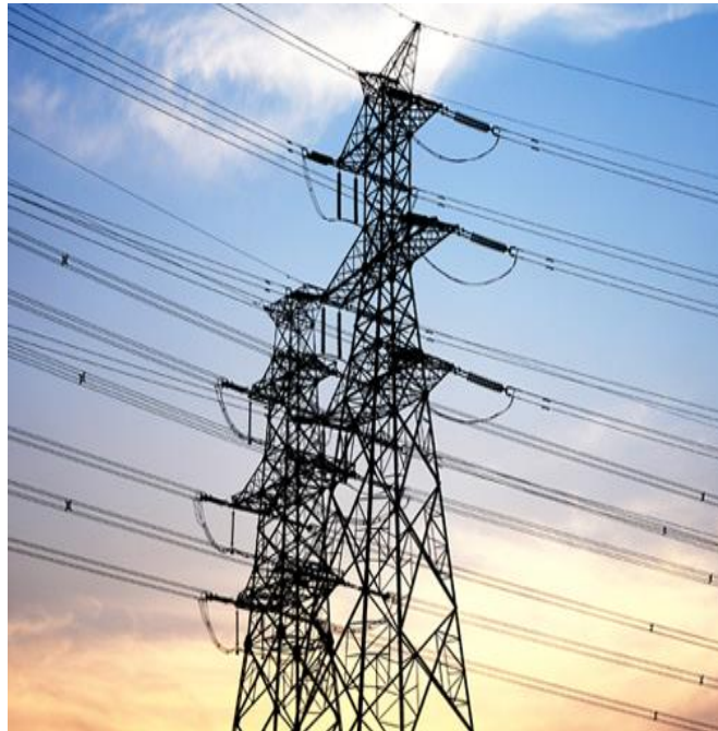
Figure 4.7 - 132 kV Transmission Line Poles
