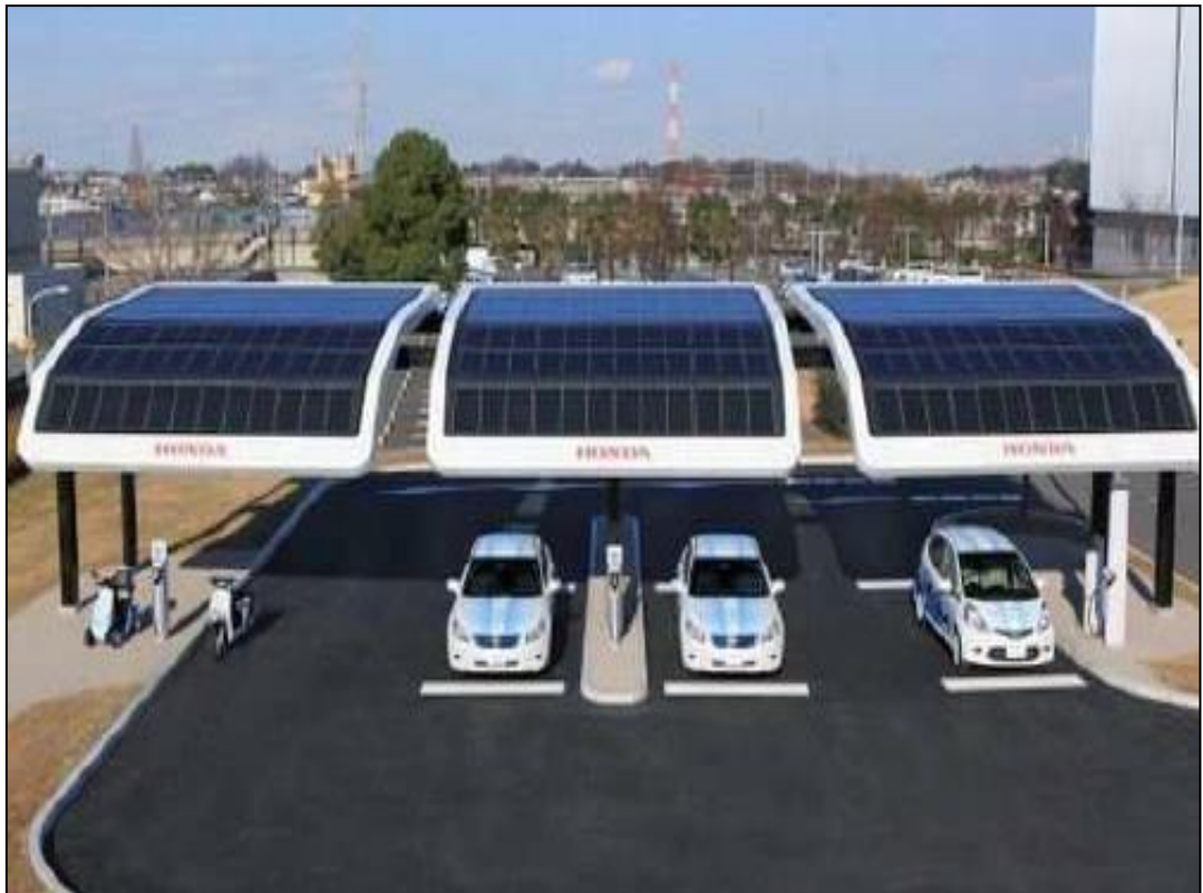
Figure 1.1: GCPV EV charging station [8]
