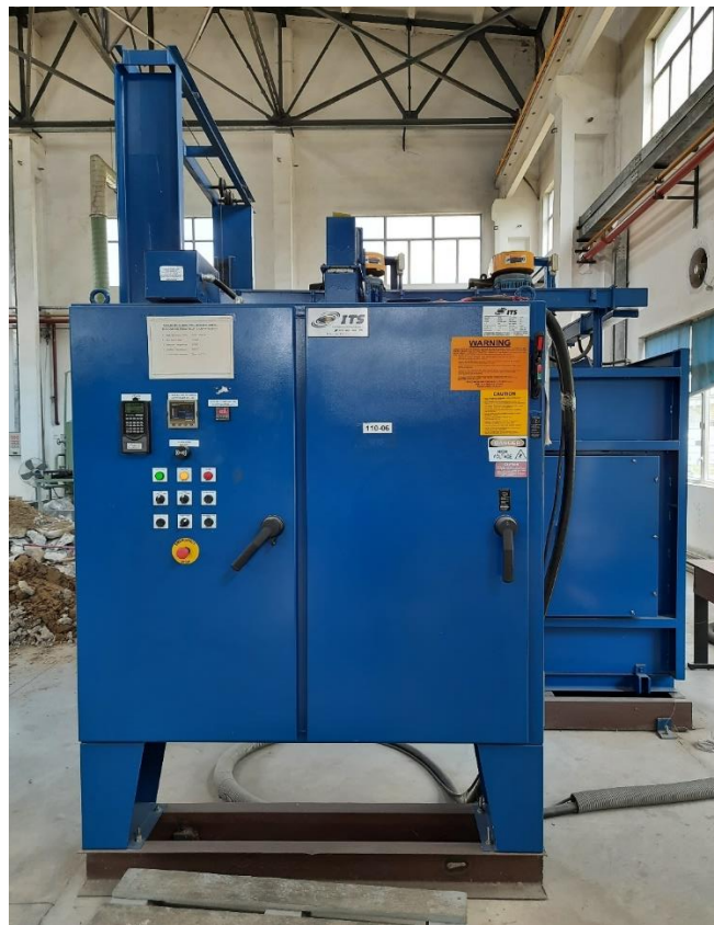
Figure 8: Box Type Air Furnace
