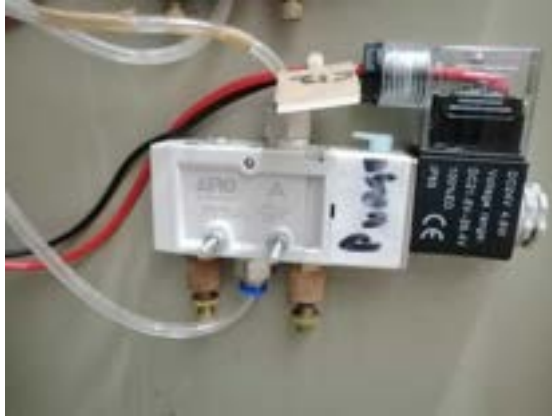
Figure 2.14: Pneumatic solenoid valve for purge
