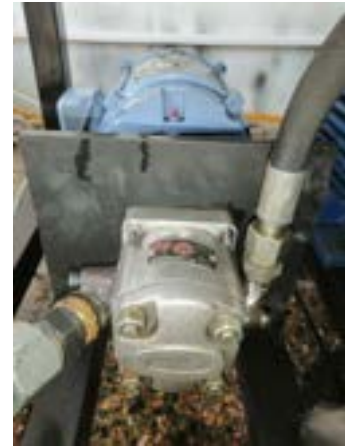
Figure 2.4: Hydraulic pump for heat exchanger line
