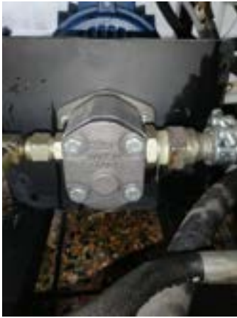
Figure 2.3: Hydraulic pump for cycling oil in complete circuit
