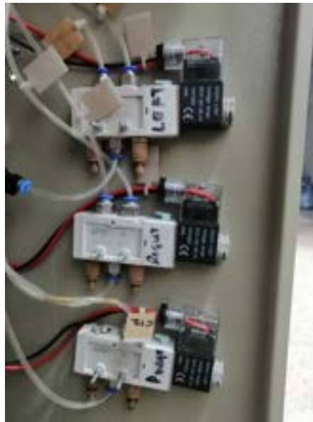
Figure 2.12: Pneumatic solenoid control valve
