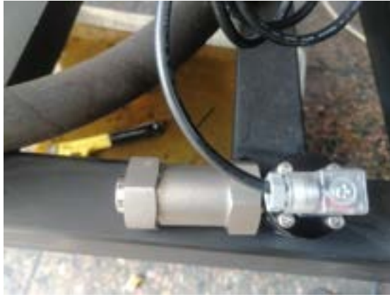
Figure 2.16: Oil flow meter
