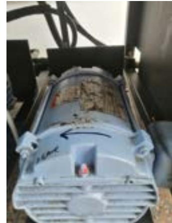
Figure 2.6: Three phase electric motor for heat exchanger pump
