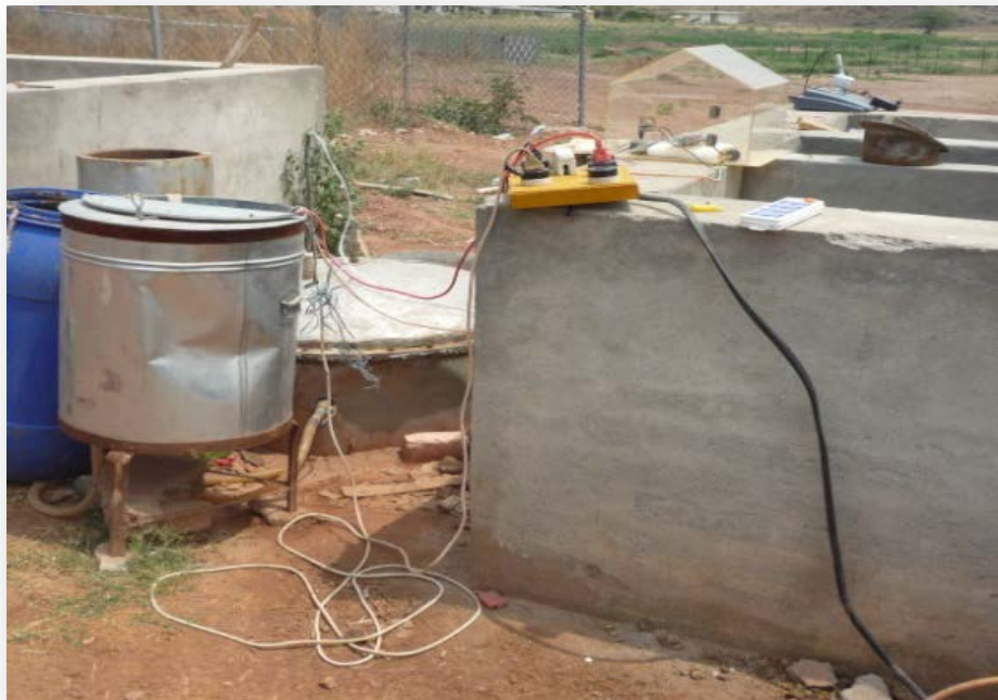
Figure 7 - Heating System for maintaining temp inside the tank
