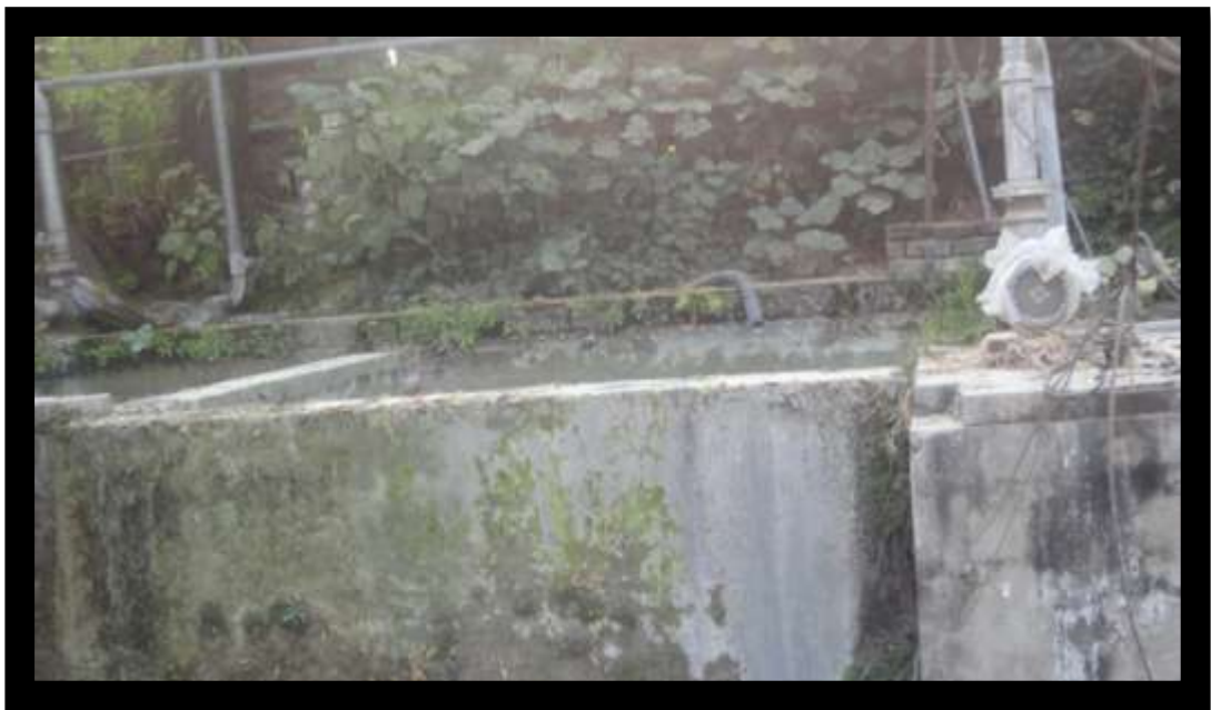
Figure 7: Water tanks used to store wastewater on site
