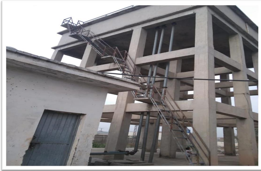
Figure 4-6 Water Supply setup in one of the labor colonies
