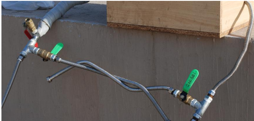
Figure 3.10: Flexible Stainless Steel Pipes
