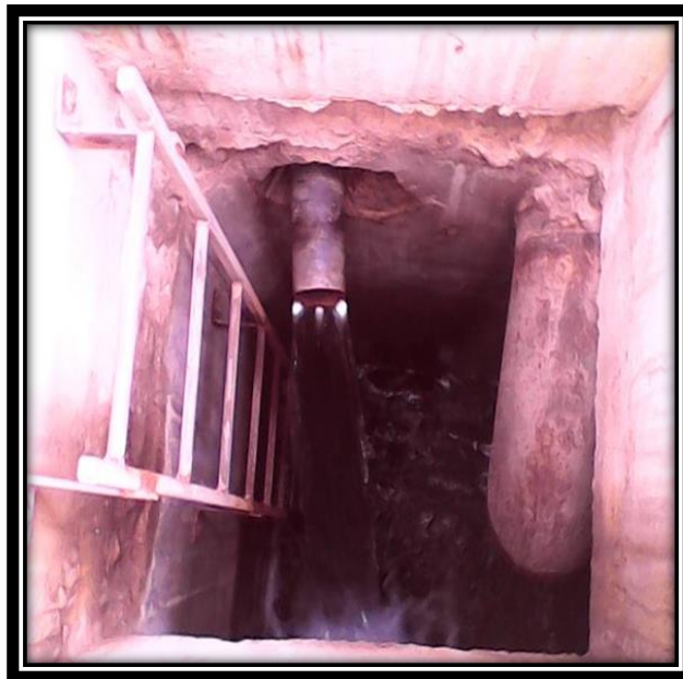
Under Ground Tank (NIT)
