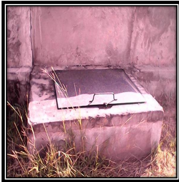
Under Ground Tank (SMME)
