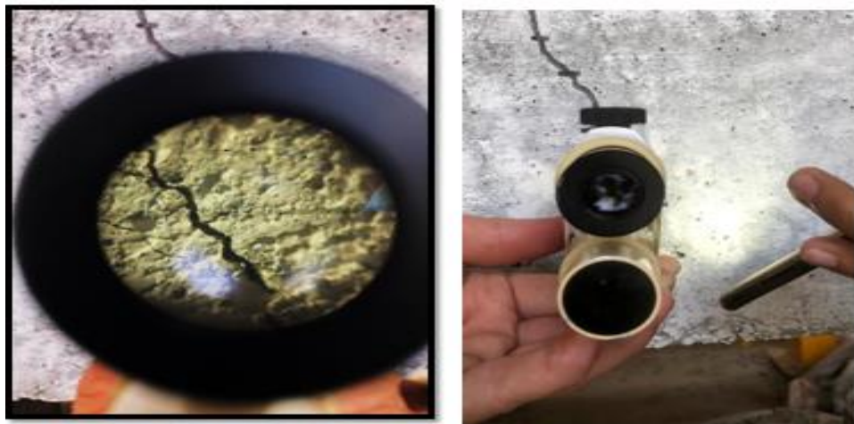
Figure 4.11 Microscope to find out crack width
