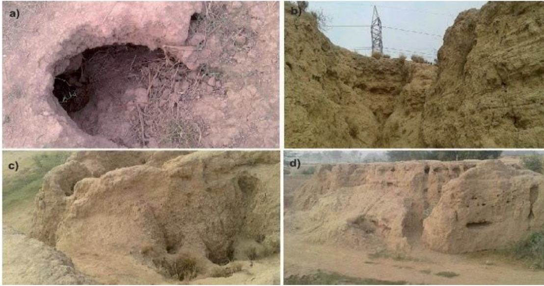
Figure 3 Soil erosion in grid station, Peshawar
