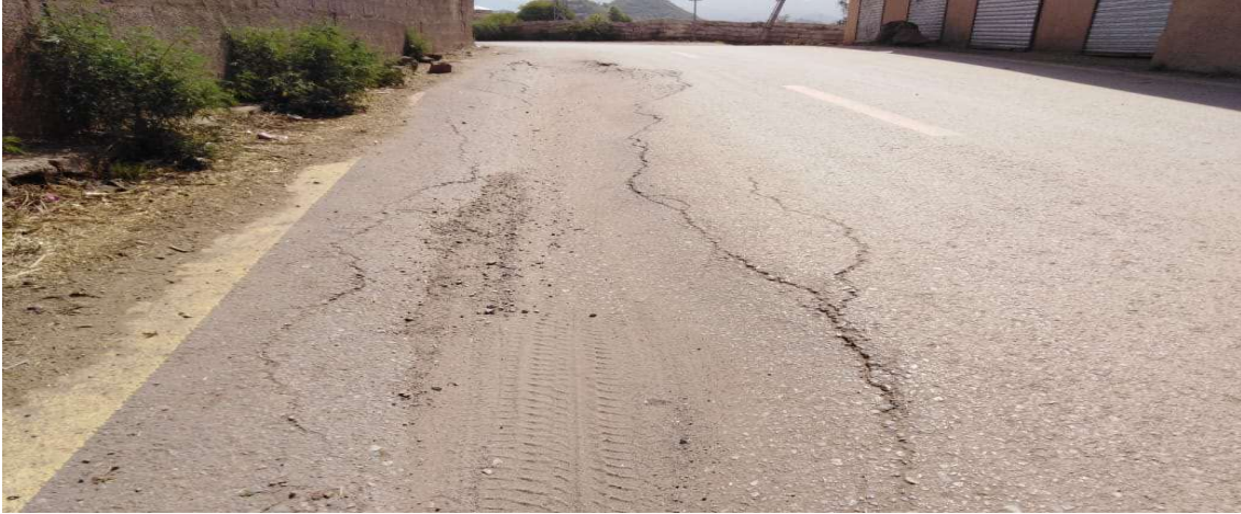
Figure 1 Settlement of road due to poor subgrade
