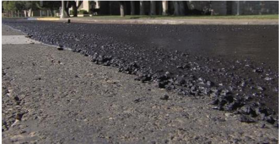
Figure 4. 2: Condition of Road after Micro Surfacing
