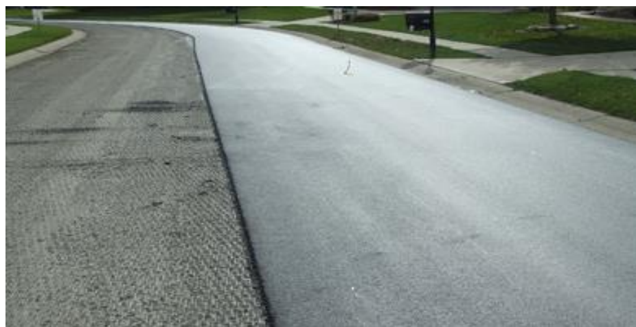
Figure 4. 6: Road after Overlay
