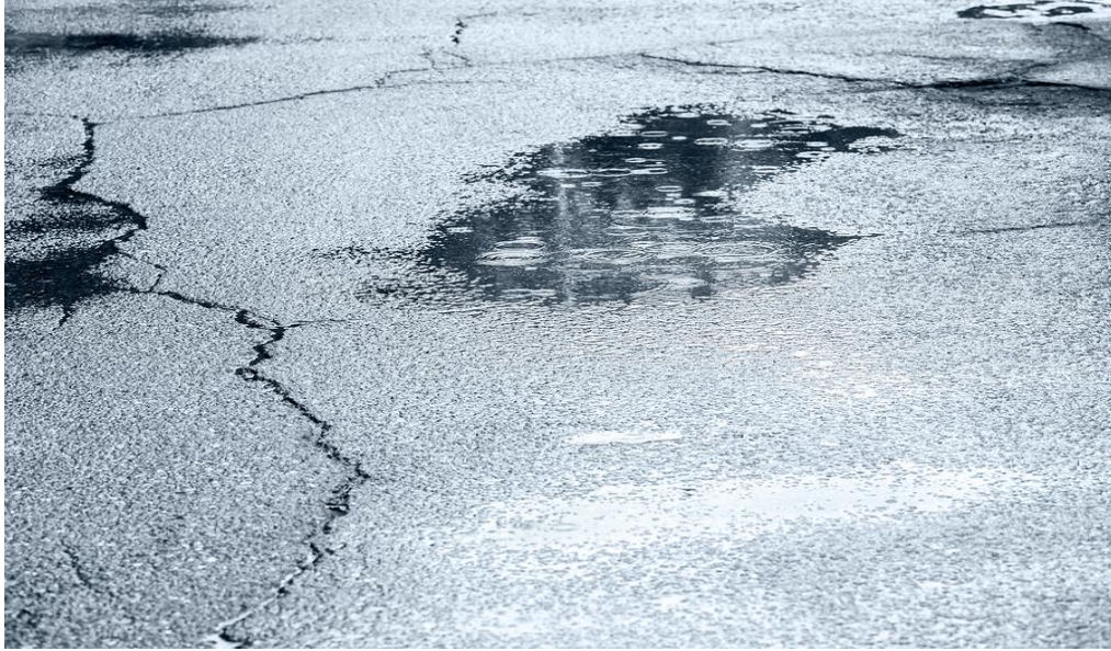
Figure with moisture damage
