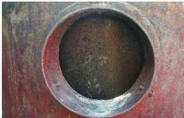
Figure 8: Corroded Tank Hole
