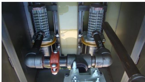
Figure 7: Hydraulic Elevator Power Unit
