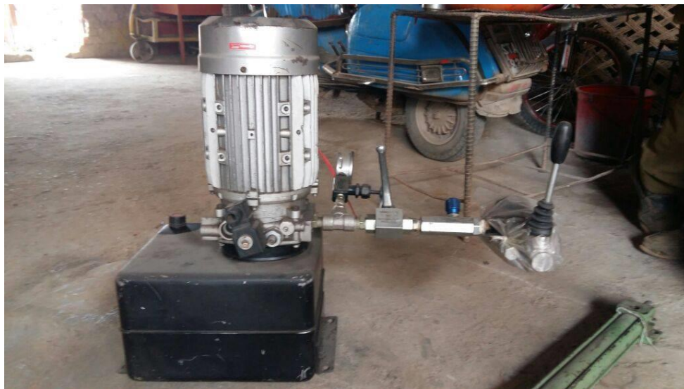
Figure 5: The motor, hydraulic pump and other components
